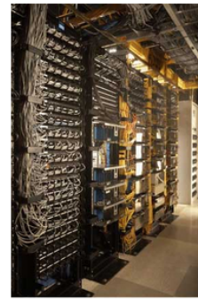
Inside Switch Data's Palo Alto data center.
